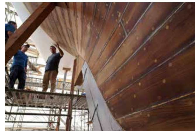
Below: External view of the Cynara , looking from the bow towards the stern, ca August, 2019. The hull surface has been carefully smoothed and polished, and then painted with an undercoating.
